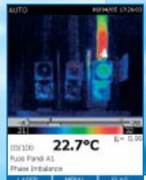
Temperature difference between phases indicates an unbalanced load.
